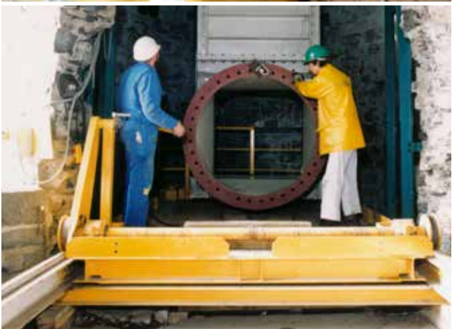
In the 1970s, an inspection tunnel was blasted into the masonry dam (see image above). The bottom outlets (centre and bottom images) were renewed in the 1990s.
