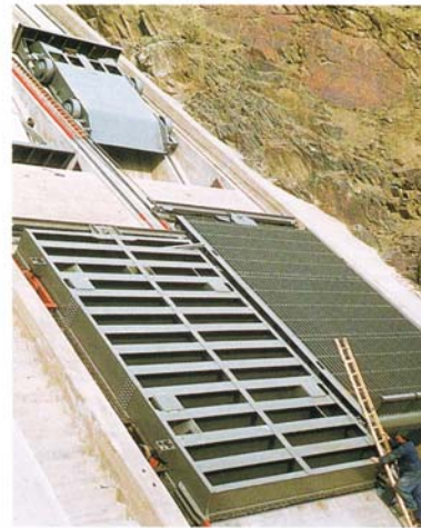
Intake of the bottom outlet with emergency gate, trashrack and shut-off unit
